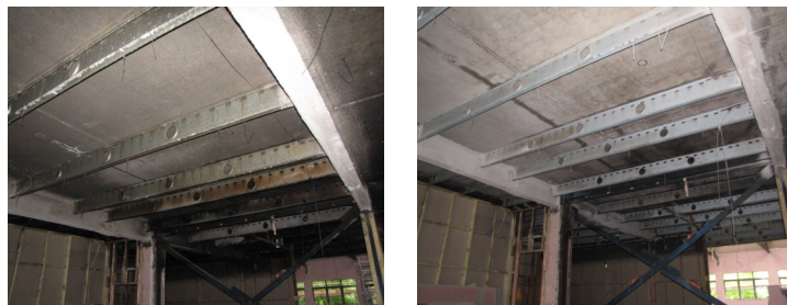
Fire damage to Glendowie Primary School. Soot, smoke and smell reduced to allow recoating of surfaces.
